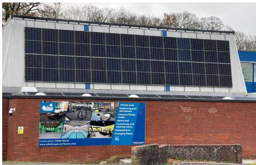
Solar panels at Calne Community Campus
