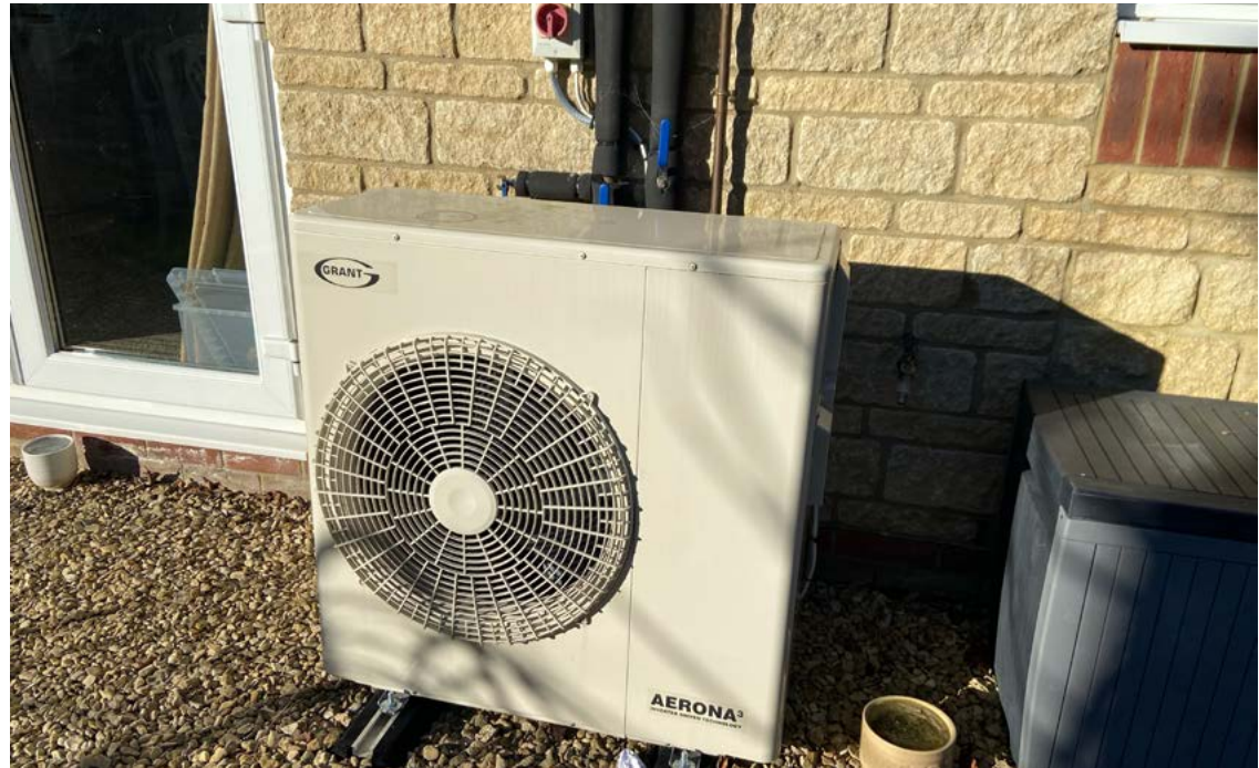
Domestic heat pump
