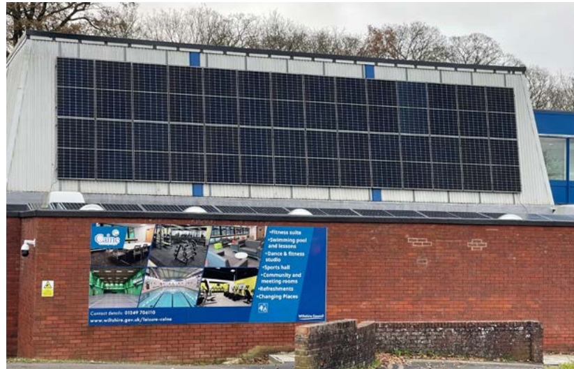
Solar panels at Calne Community Campus
