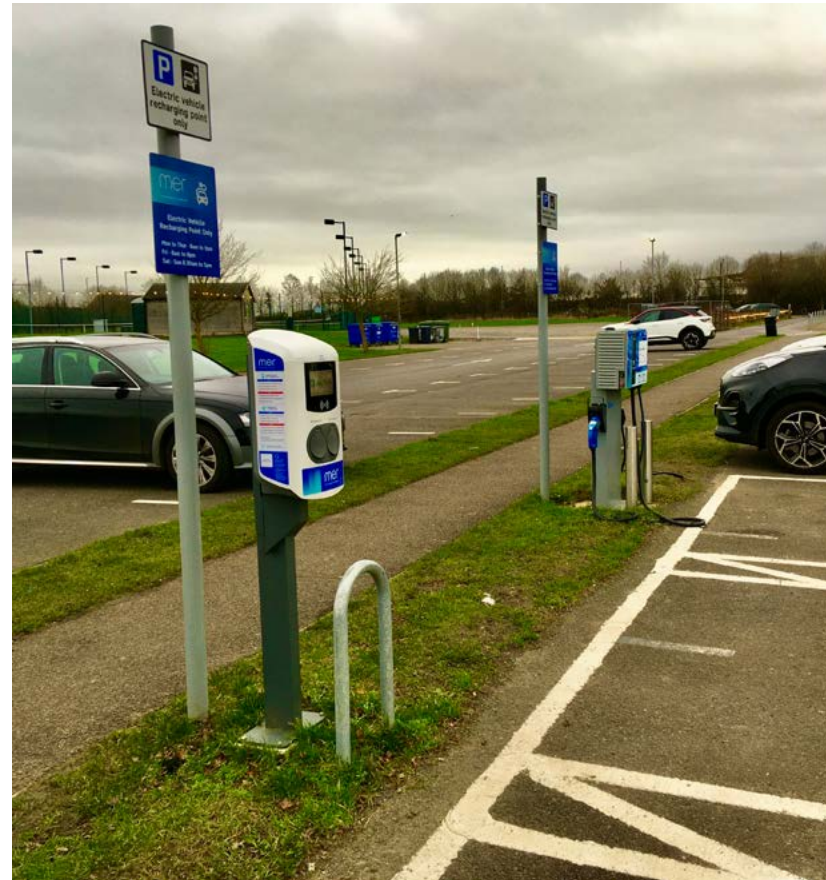
Charging points at Beversbrook Sports Centre
