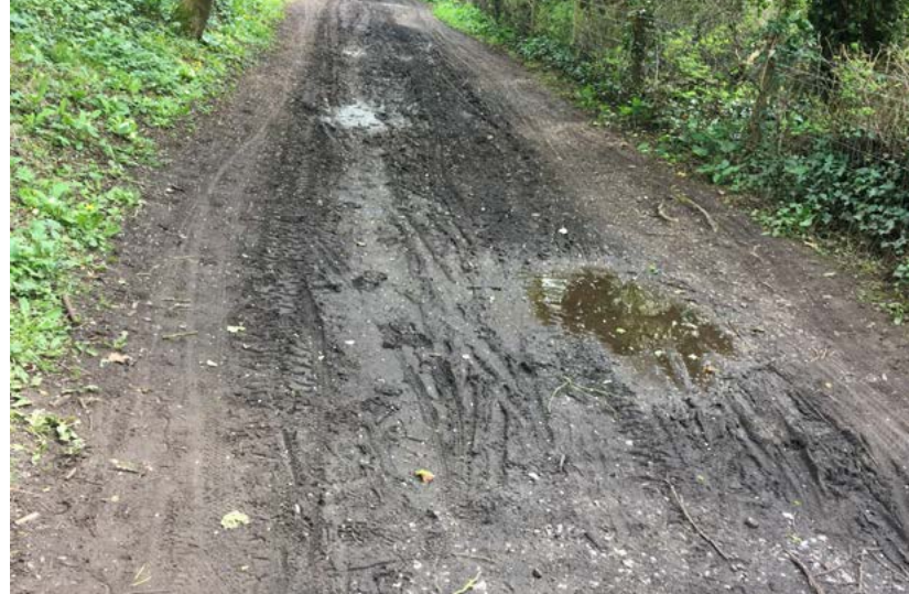
Cycle track between Calne and Studley showing poor surface
