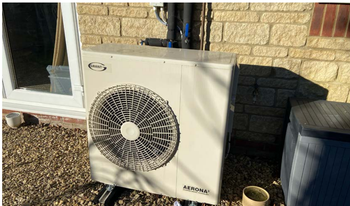
Domestic heat pump
