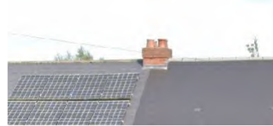
Solar panels installed on grey slate roof with red brick chimney
