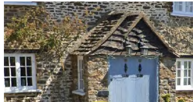
Gabled porch with dark coloured slate and black weatherboarding at the front
