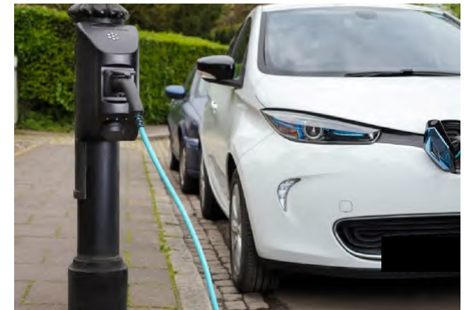
Figure 115: Example of on-street electric vehicle charging points.
