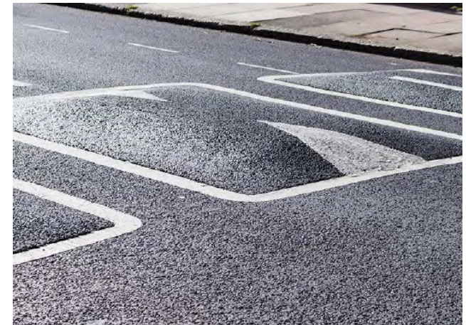
Figure 100: Example of a speed cushion.
