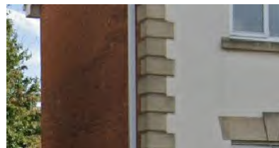
Beige render with Bath stone dressing and red brick on the side
