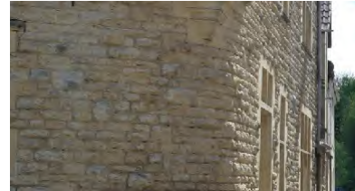
Exposed rubble on façade
