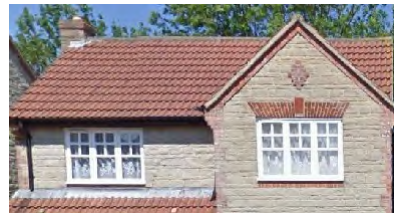
Red clay pantile gabled roof with chimney, local Bath stone façade with red brick dressing
