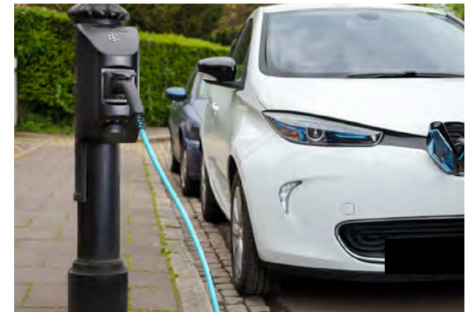
Figure 115: Example of on-street electric vehicle charging points.
