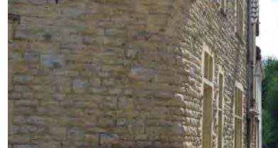
Exposed rubble on façade
