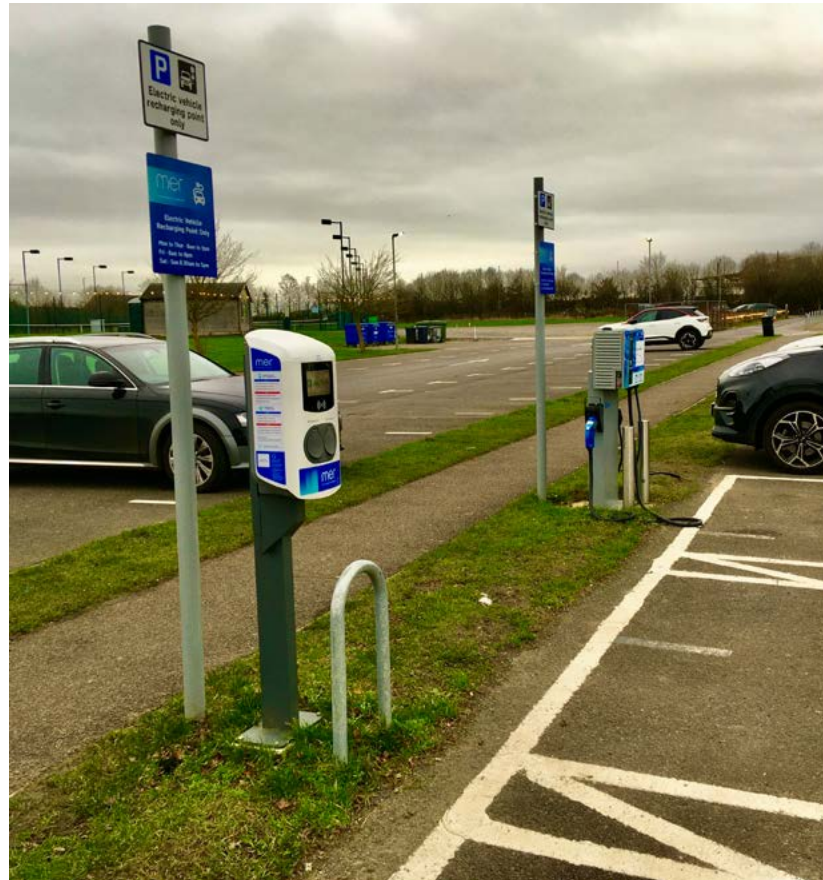
Charging points at Beversbrook Sports Centre
