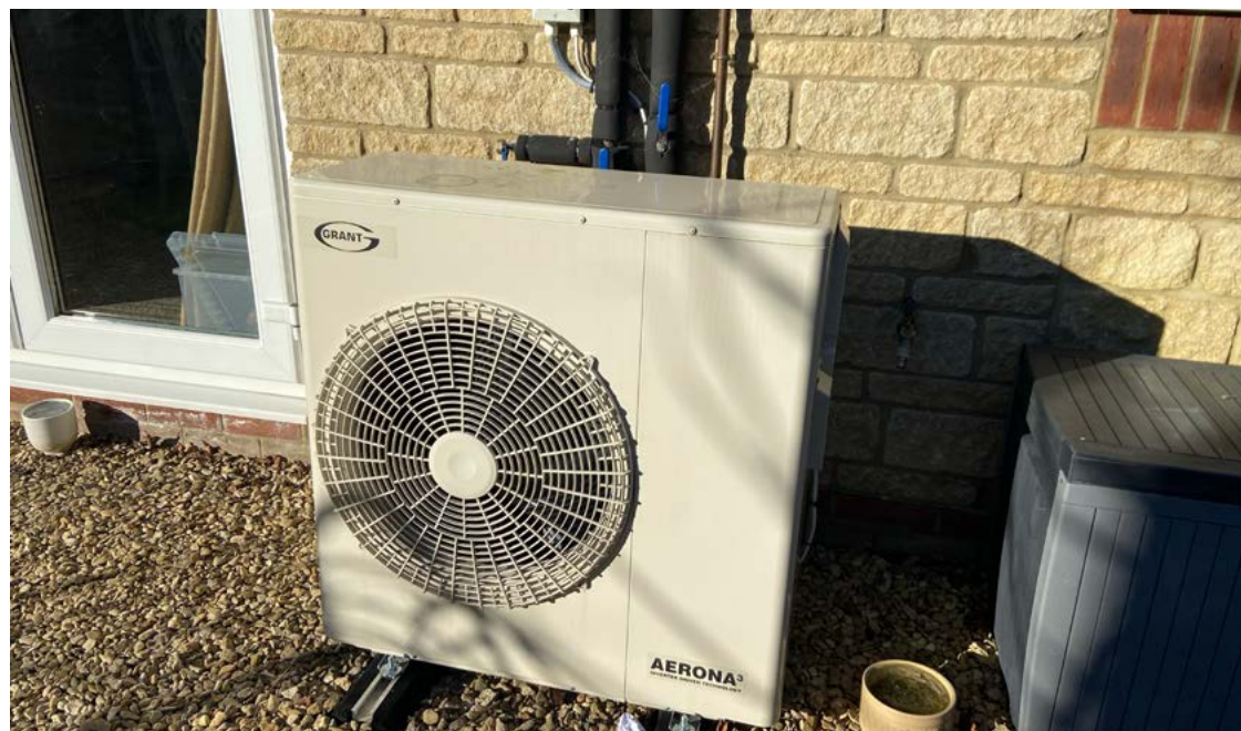
Domestic heat pump
