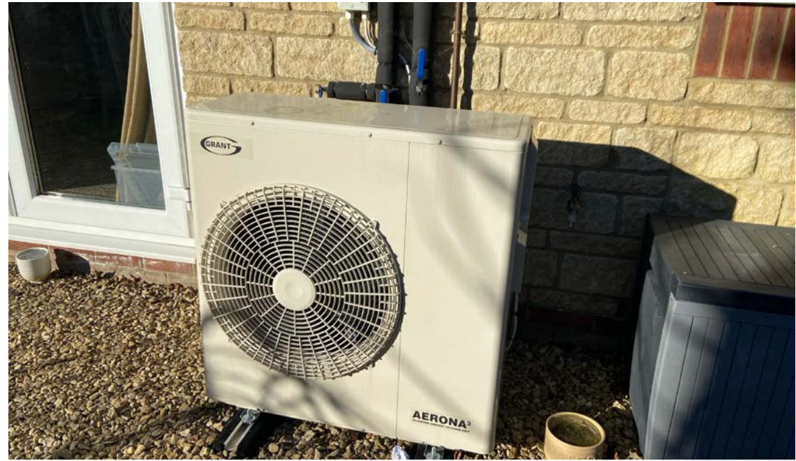
Domestic heat pump
