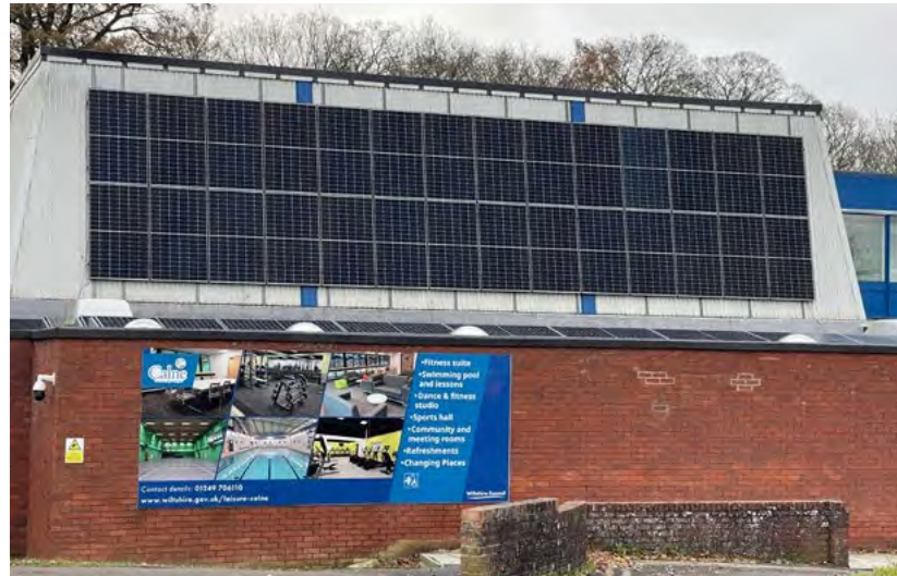
Solar panels at Calne Community Campus
