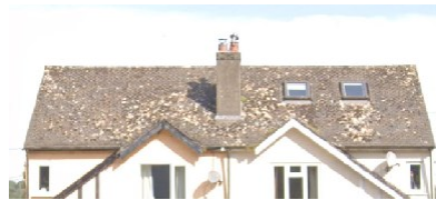
Double gabled roof with clay tiles and skylights, white-rendered façade with black timber frame
