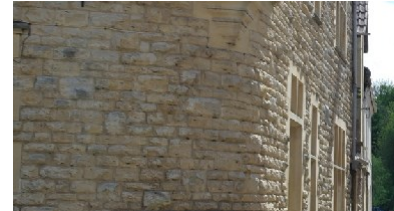
Exposed rubble on façade
