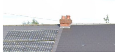
Solar panels installed on grey slate roof with red brick chimney
