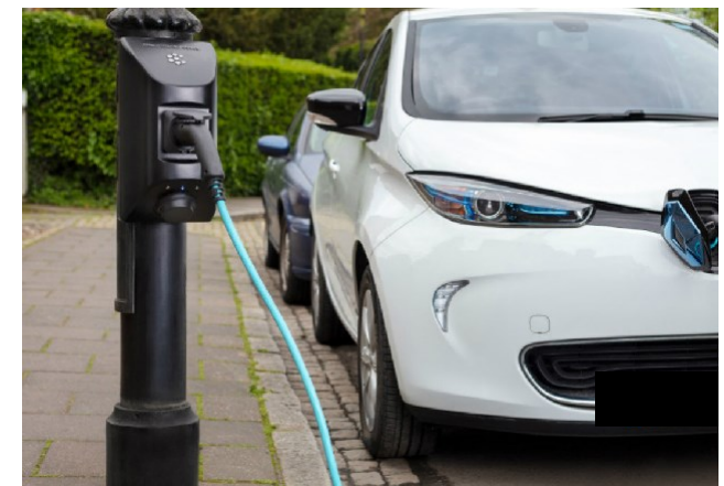
Figure 115: Example of on-street electric vehicle charging points.
